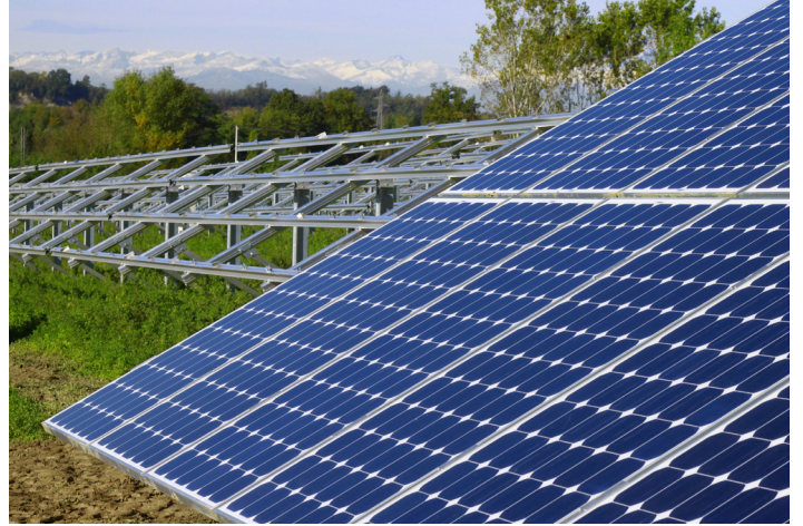
Steel construction for PV-sites
